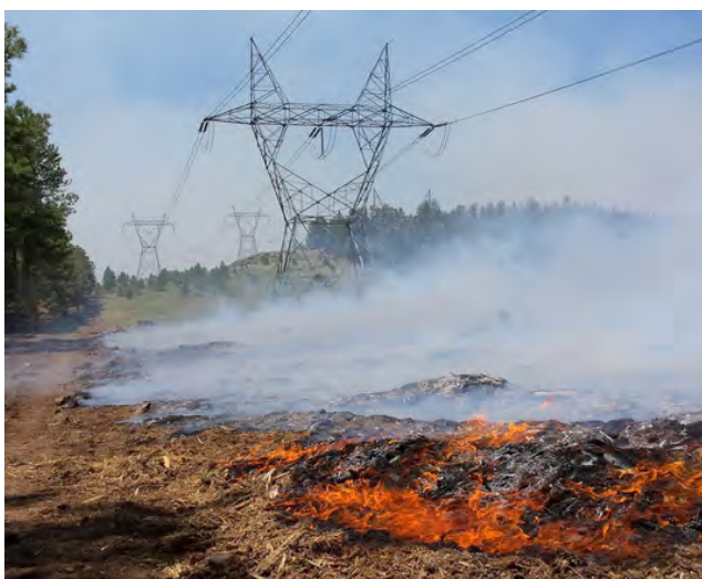
Wildland fires encroach on high power lines during a 2015 fire in the Coconino National Forest (Image Source: Liza Simmons/USFS)
